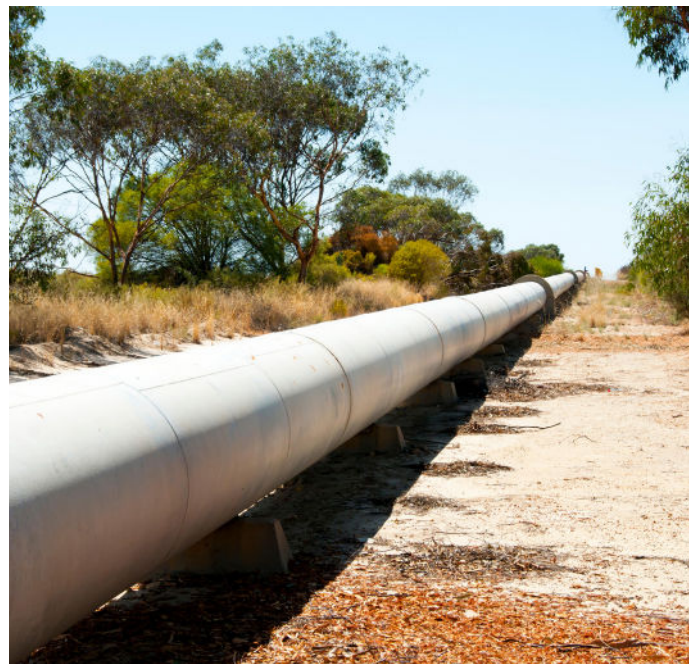
Image: Example of an aboveground water supply pipeline.
