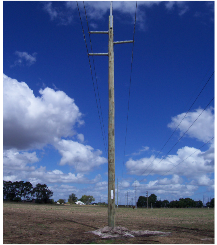
Image: Example of a 132kv single pole powerline.
