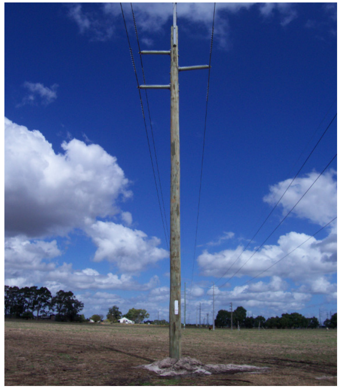
Image: Example of a 132kv single pole powerline.
