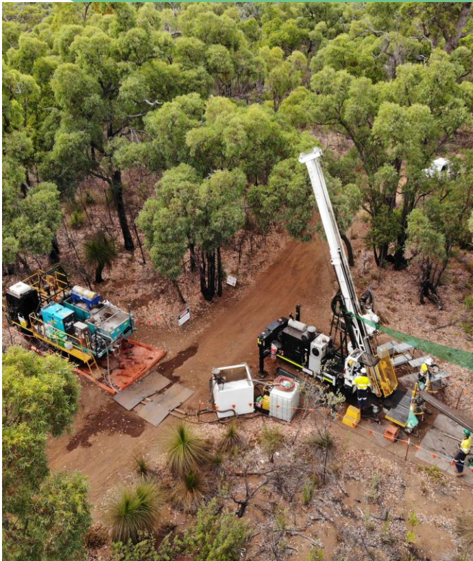
Chalice's compact drill rig operating on existing access track in the Julimar State Forest.
